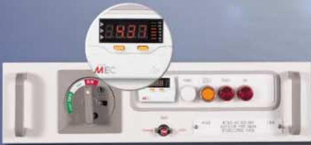
*Fig. (D-EMPR in the MCC unit)
